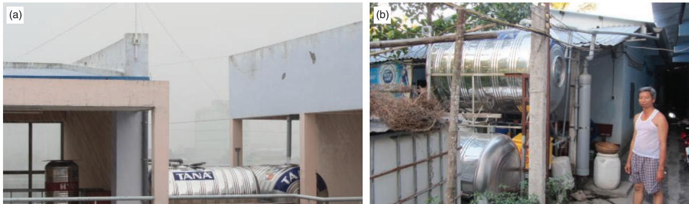
Case Study 14.1 Figure 6 Demonstration of rainwater harvesting systems for safe water supply: One pilot system on Can Tho University campus for research and testing water quality, and one at a peri-urban household in Le Binh ward, Cai Rang District, for reality check.
