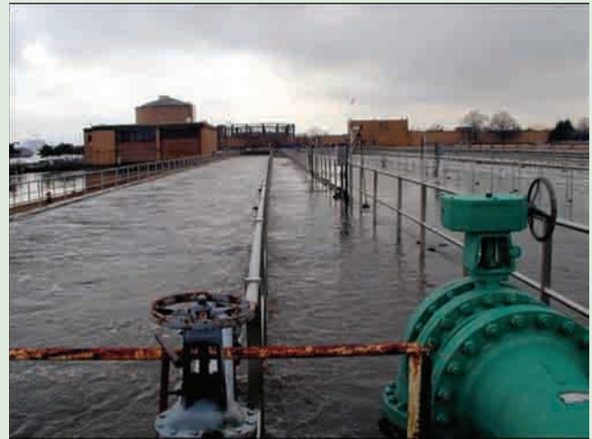
Box Figure 5.13: Flooding at a coastal water pollution control plant (WPCP) in New York City.
